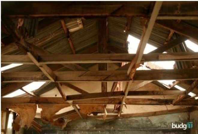
Methodist high school with broken roof
