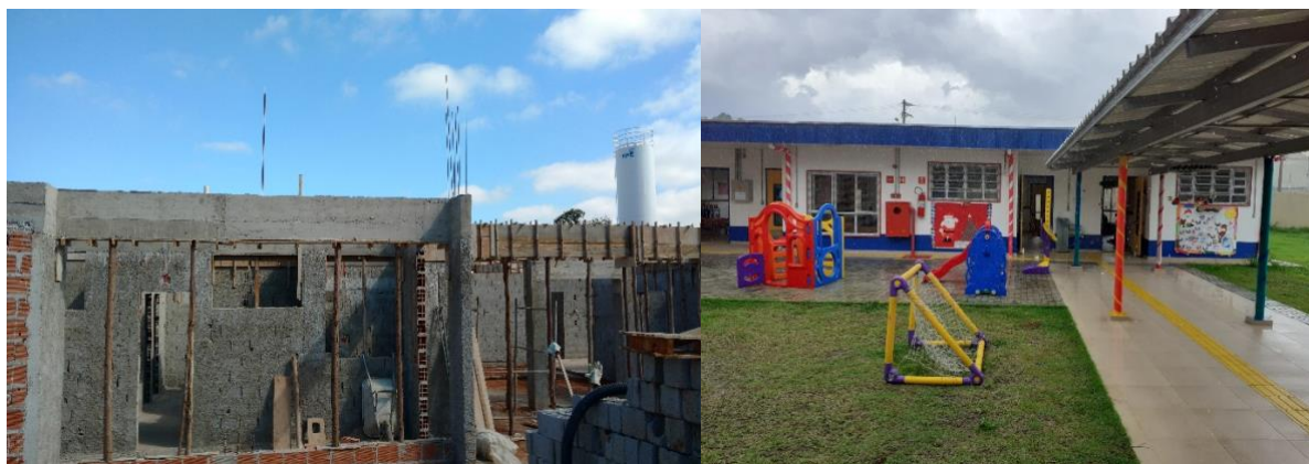
Picture 2 and picture 3 - Nursery Construction monitored by CSO Taubaté (it was paralysed at the beginning of the project and was delivered during project implementation).
